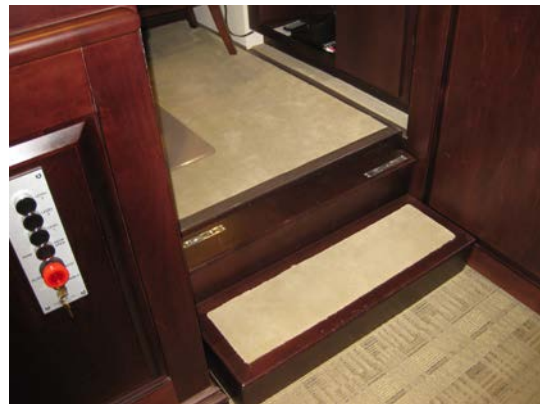
Electronic Lift at Judge's Bench, Isle of Wight Courthouse
