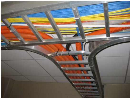
Communications Room Cable Trays Fairfax County Courthouse
