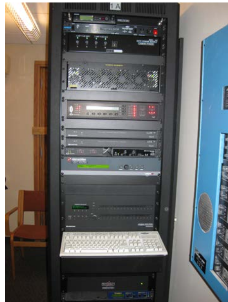
Dedicated Courtroom AV Closet, Fairfax County Courthouse
